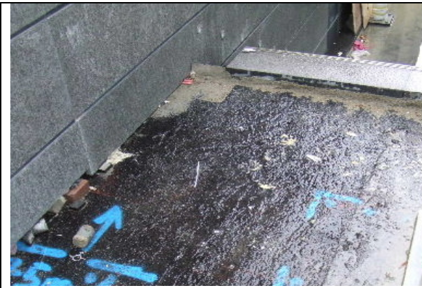
7. A gutter down the left edge of the stairs which contains drainage cell material under the tile, will see water from the landing take that pathway and stop it from emerging through the stair risers.
