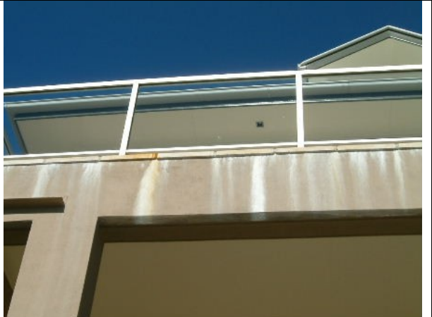
6. Where the gradient in the substrate leads to a free edge, efflorescence will form on the riser. To avoid this problem have a “waterstop” angle sealed to the floor at the edge or 1 tile in from the edge, and have the substrate behind the angle graded to a drain.
