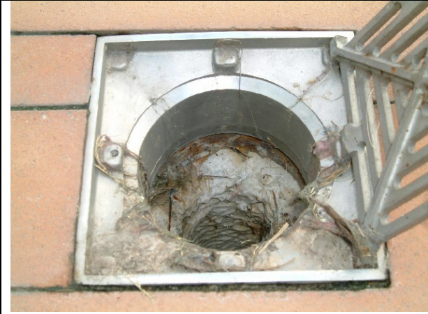
5. When the drain is open at the neck, and there is a gradient in the substrate to the drain, the efflorescence forms down the drain pipe and not on the tiles.
