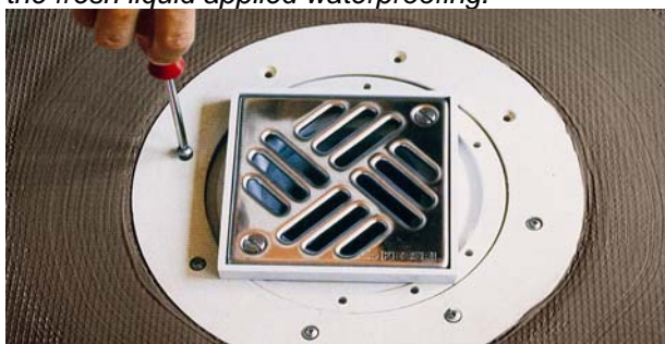
Image 3: Bolting of the fixed flange after coating of the waterproofing gasket with liquid applied waterproofing material
