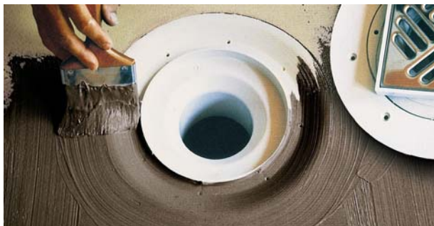
Image 1: Coating of the fixed flange with subsequent fitting of the waterproofing gasket into the fresh liquid applied waterproofing.
