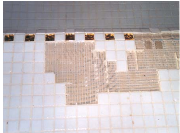
Image 10: Mesh mounted Mosaic must not be used in permanently wet and underwater areas, since this can rapidly lead to cavities and detachment of the mosaic pieces (hydrolysis of the adhesive!).
