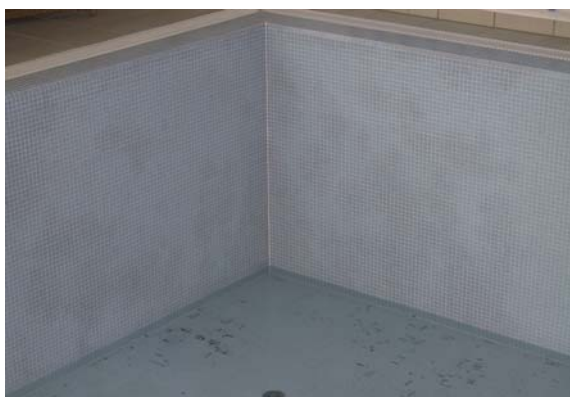
Image 11: In the case of translucent mosaic in particular, laying and grouting must be carried out using epoxy resin in order to prevent cavities.
