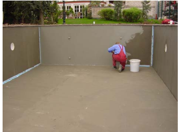
Image 5: Subsequent coating of the waterproofing tape with a second coat of liquid applied waterproofing.
